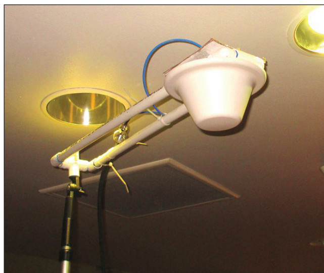
Figure 8. Indoor antenna on mast performing PIM survey test
