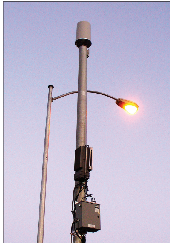
Figure 9. Small cell antenna installation
